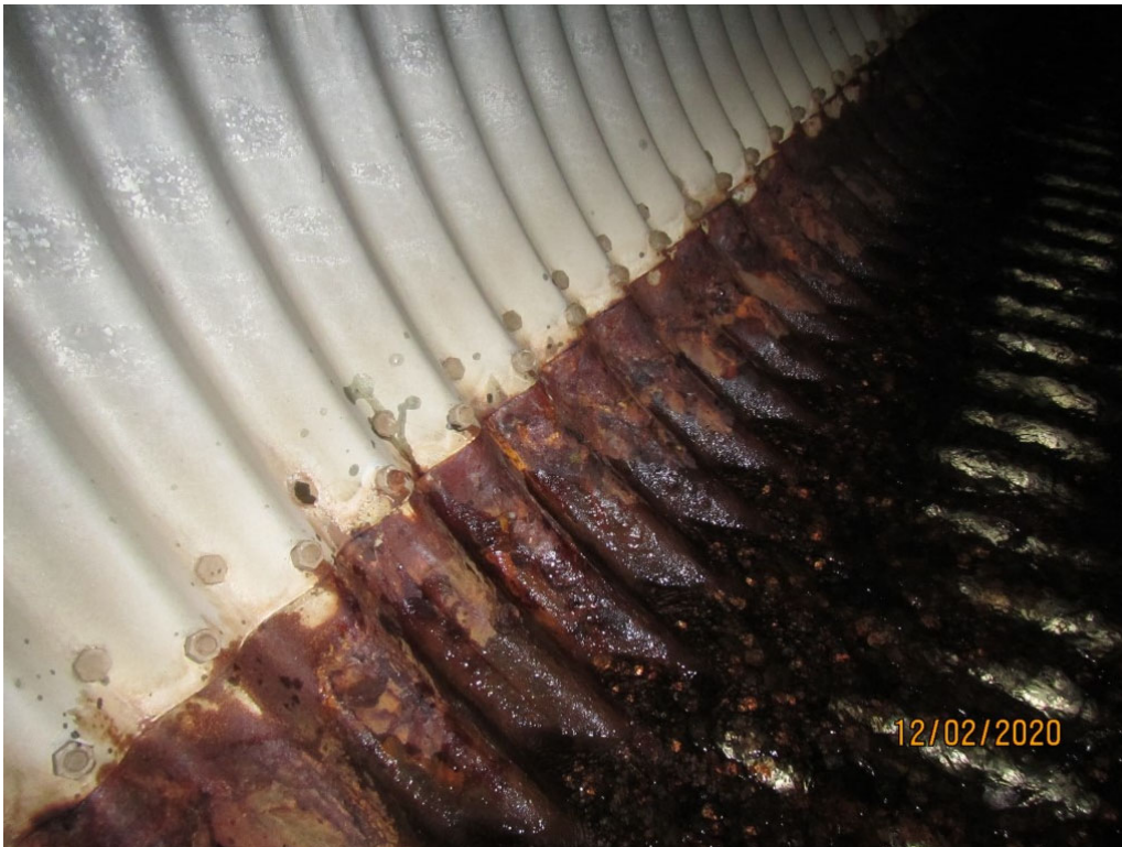
Picture 7: Rusted invert
